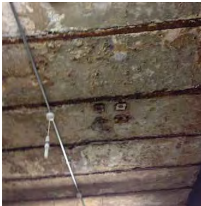
Figure 4.2 – Slab soffit showing evidence of dampness
