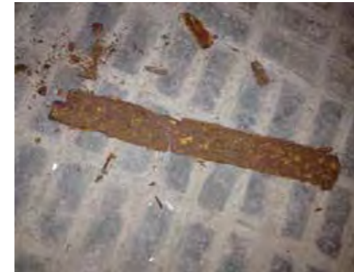
Figure 4.2 – Delaminated bottom flange of filler joist
